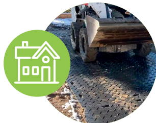
Residential Contracting Water, Gas Electricity, Powerline, Landscaping
